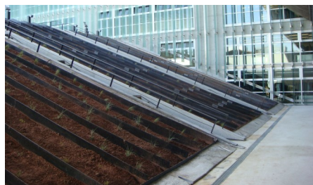
In the pitched roof area Georaster®-elements have been applied to hold the substrate.
